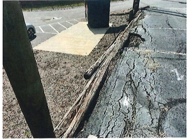
Figure 9: Damaged asphalt on upper parking lot.
