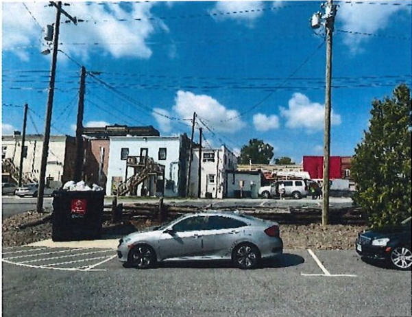
Figure 2: Looking northwest at end of wall near dumpster pad. This is the high end of wall.
