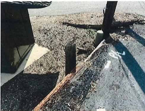
Figure 7: Utility poles and phone service at base of retaining wall near dumpster.
