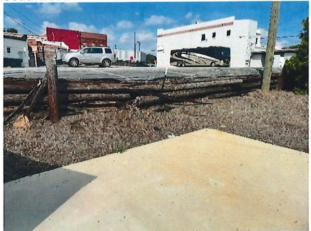
Figure 4: Retaining wall near dumpster pad.
