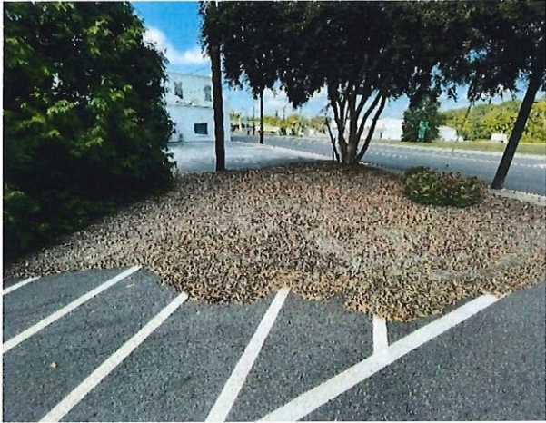
Figure 6: Upper end of both parking lots. No retaining wall.
